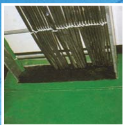
For Cable Tray(slab)
