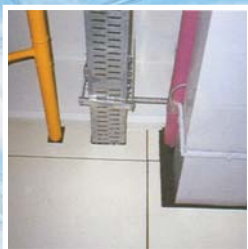
For Pipe and Duct Way
